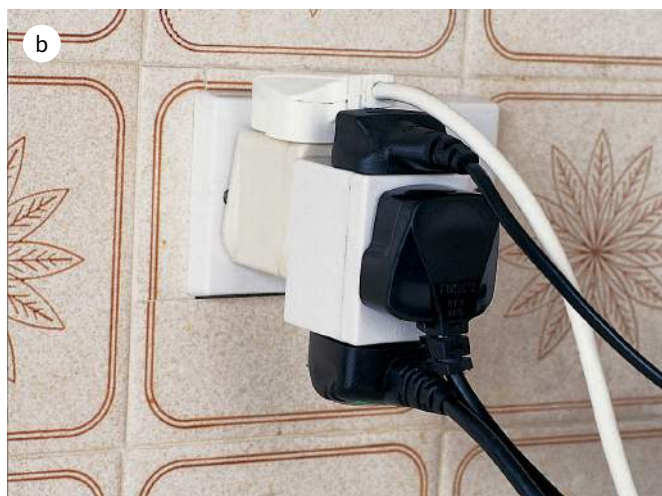
Figure 10.19 a Correct use of an electrical socket. b Here, too many appliances (resistances) are connected in parallel. This reduces the total resistance and increases the current drawn, to the point where it becomes dangerous.
