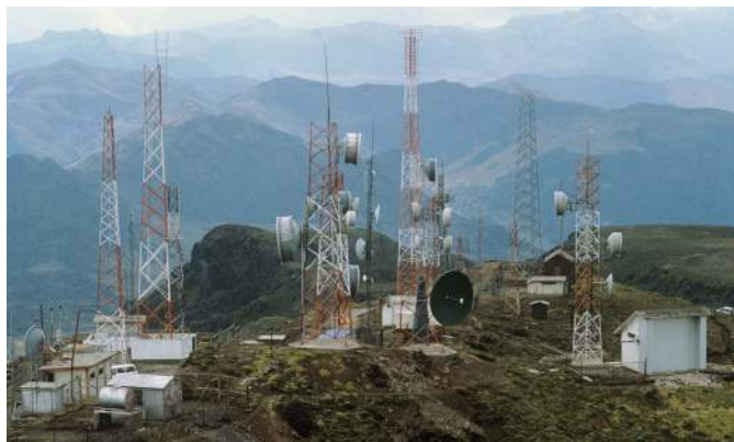
Figure 13.13 These telecommunications masts are situated 4500 metres above sea level in Ecuador. They transmit microwaves, a form of electromagnetic radiation, across the mountain range of the Andes.
