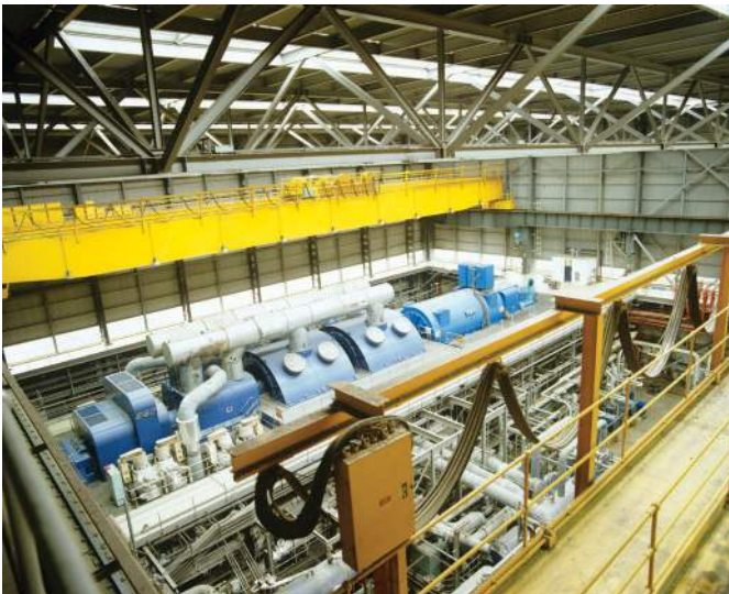
Figure 29.3 Generators in the generating hall of a large power station.
