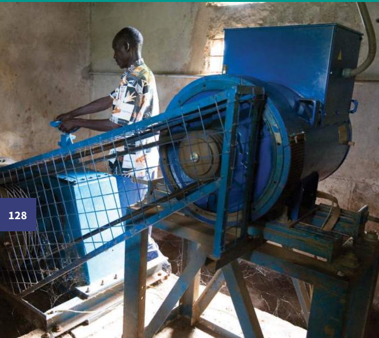
Figure 9.1 An operator controls the water inlet at the Kabiri Falls power plant. The generator is on the right.
