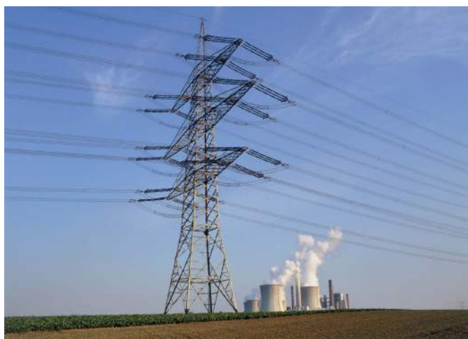
Figure 9.16 A power station and electrical transmission lines. How much electrical power is lost as heat in these cables? (See Worked examples 6a and 6b.)
