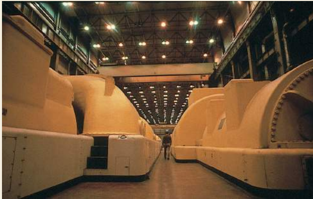
Figure 28.15 The generators of this power station produce electricity at an induced e.m.f. of 25 kV. For Question 6.
