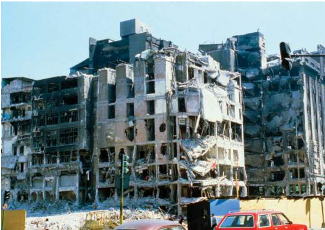
Figure 19.33 Resonance during the Mexico City earthquake of 19 September 1985 caused the collapse of many buildings. The earthquake, whose epicentre was in the Pacific Ocean, measured 8.1. Many lives were lost.
